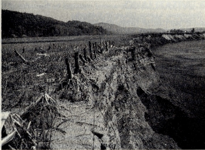
Figure 6: Scouring of river bank.
